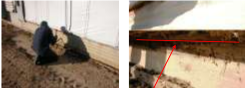
Crack between wood sill and concrete foundation.
