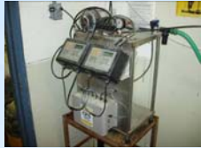
Central Fogging System
