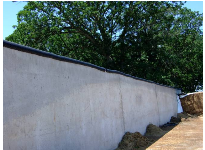
Figure 2. Plastic drain pipe used to cover the top of the wall to prevent side wall plastic from being torn or punctured.
